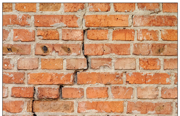
Figure 28: Example 2 of Damaged Brick
