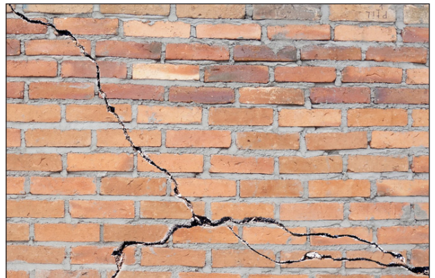
Figure 27: Example 1 of Damaged Brick
