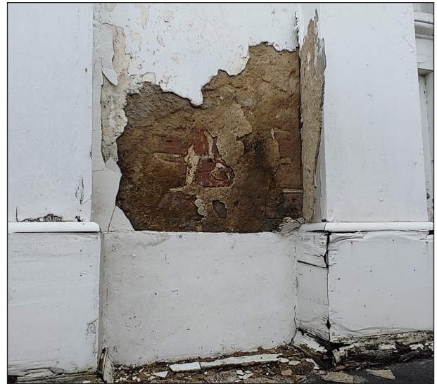
Figure 29: Example of Damaged Stucco 1
